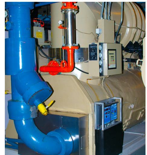
This recent medical center project included the installation of new, more efficient chillers and a new building control system that automates and optimizes the chiller plant.
